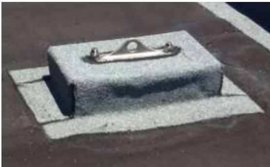
D. The hobs are water proofed with membrane (different anchor model shown AA408)
